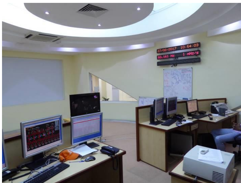
Television in center displays the current grid's diagram. The operators in the cockpits are supervising the grid condition. The clock, frequency and display enabling to display the fault messages are set on the wall
